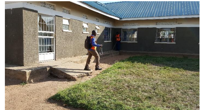
The affected Maternity Block at Avogera Health Centre
